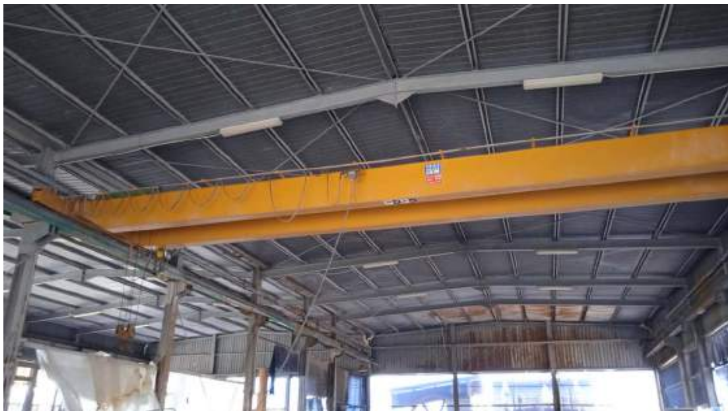
4. Carroponte 5 tonnellate Pellegrini
